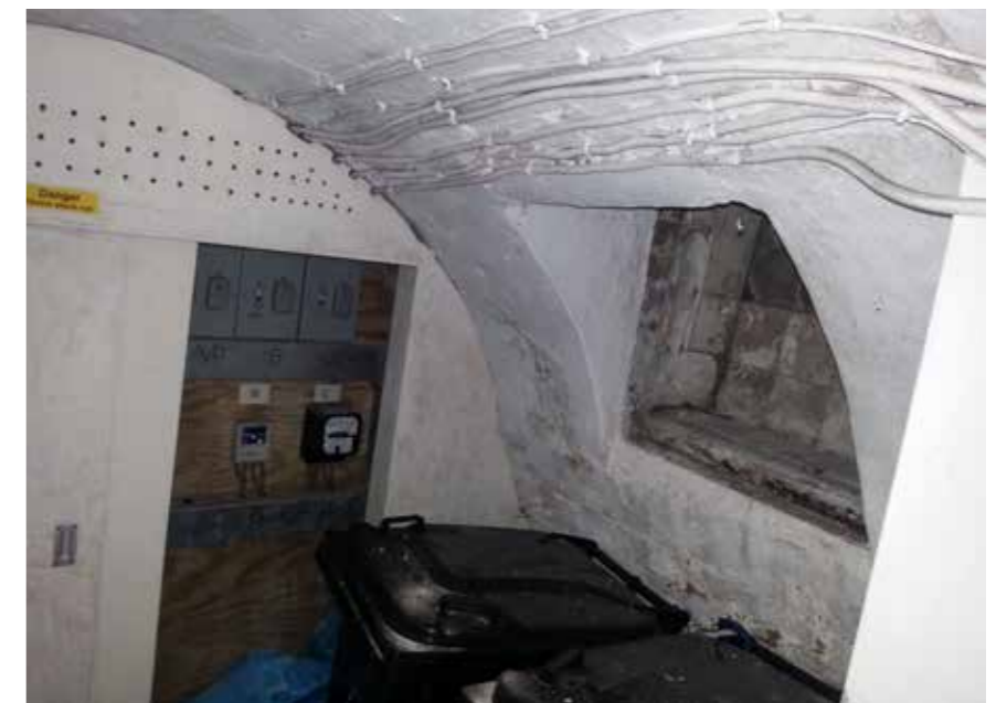
Existing services store
