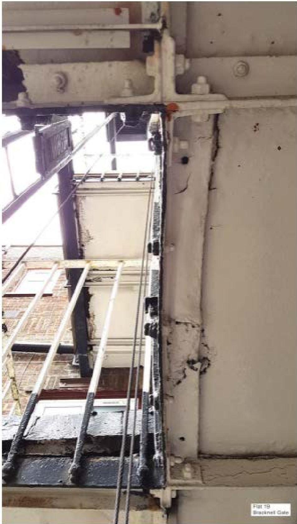
Figure 1 – Failure of the Lintel
