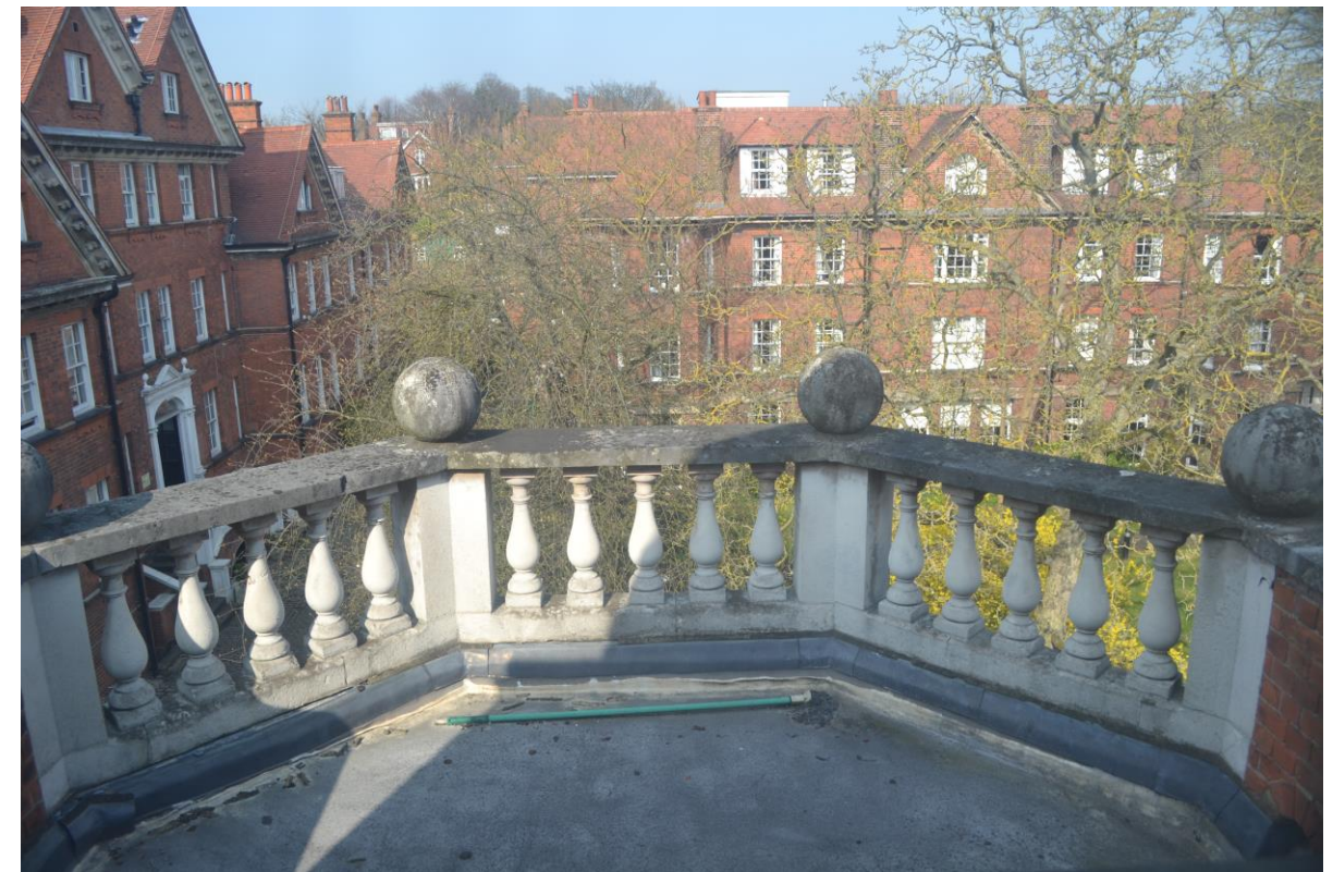
Figure 90. The balcony at the second floor level to the rear of the former Skeel Library.
