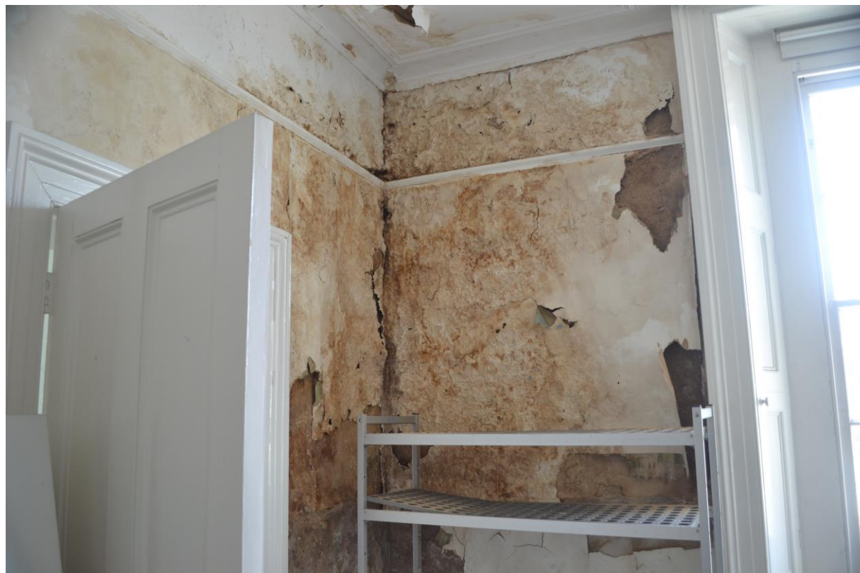
Figure 68. An image of the damage caused by water ingress at the first floor level.
