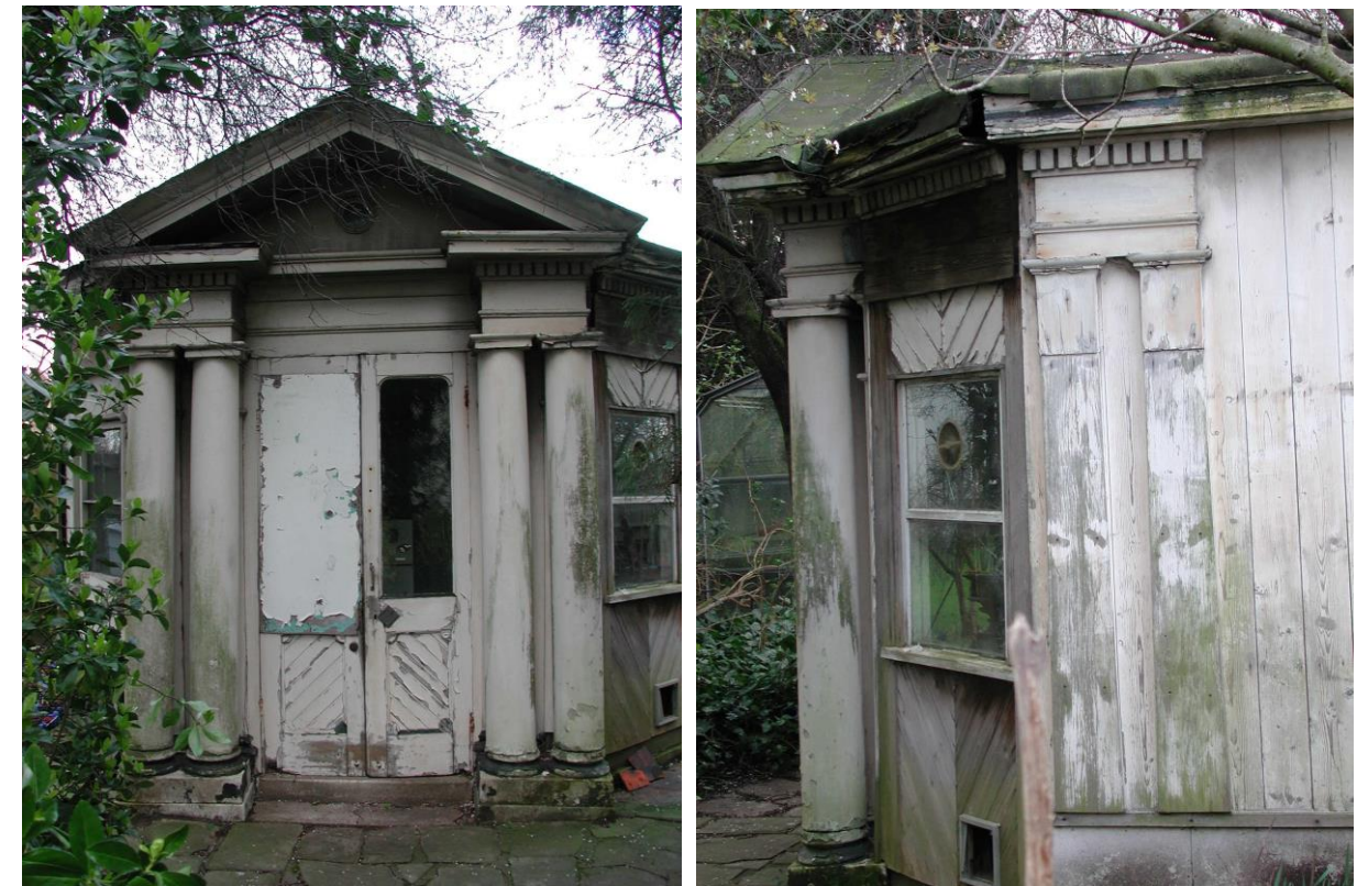
Figure 71 A photograph of the Summerhouse taken in 2002. These give an indication of the physical state of the building 13 years ago.
