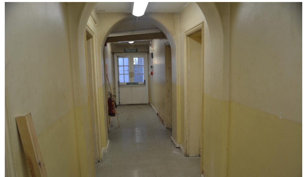
Figure 67. A photograph of the corridor at the basement level of Kidderpore Hall. The interiors at the basement level are, as one would expect, utilitarian in character and reflect their function as the original service areas of the residence.
