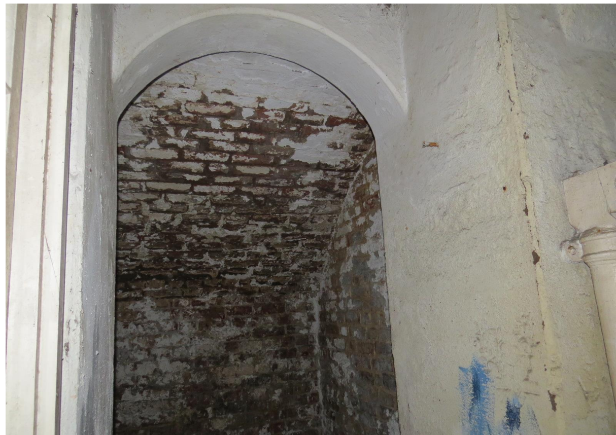
Figure 64. A photograph of one of the vaults at the basement level of Kidderpore Hall located underneath the pavement.
