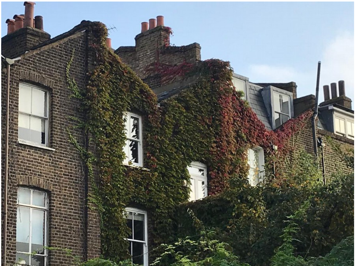
View of the rear facades to Falkland Road showing butterfly roof and gable walls.
