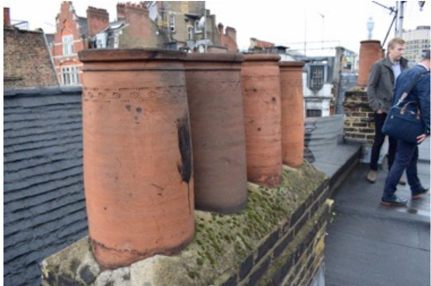
Roof-level view, looking southwest, showing ceramic chimney pots – indicative of a late 19th century date for the added fourth floor.
