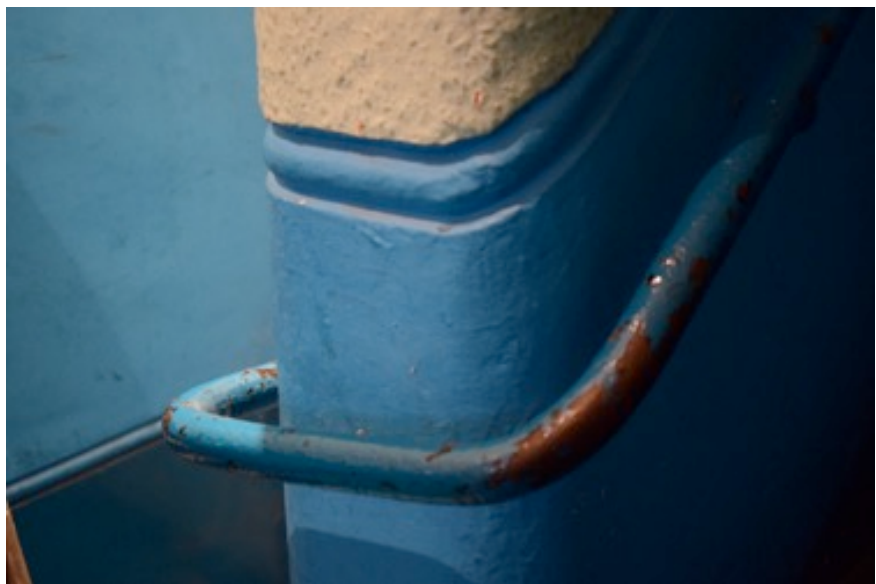
Detail of staircase, rebuilt in first half of 20th-century to enable private, fire-resistant access to individual offices (replacing what was originally wood stairs rising up the rear rooms of the each floor of No. 5)
