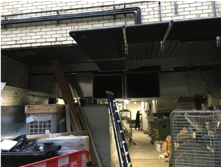
1 – Ductwork located within service bay – sits within building enclosure
