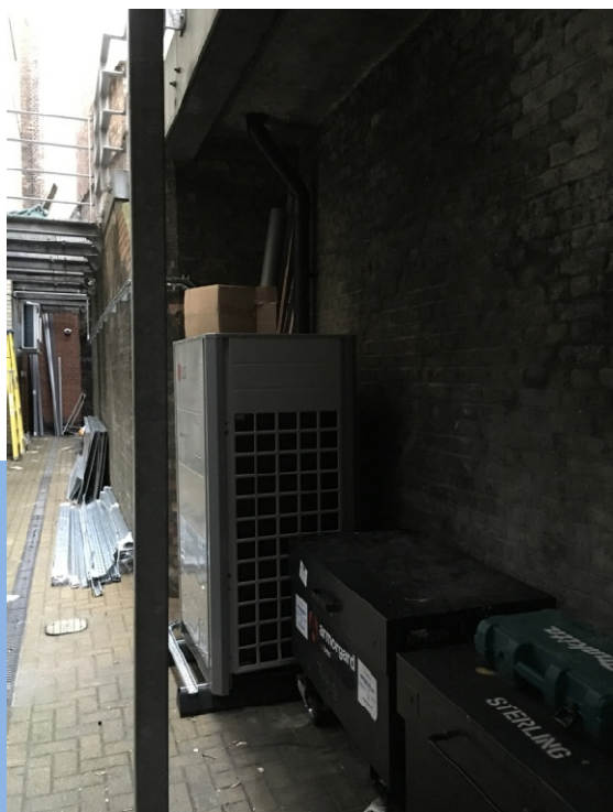
4 – units concealed within wall reveal
