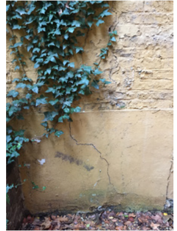
Figure 52 : Cracks & damage to party wall between no. 4 & no. 2 Chalcot has
