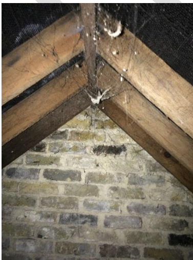
loft space of building 1 – heavy cobwebs within ridge space
