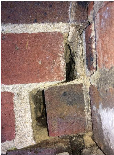
ingress with cobwebs noted
