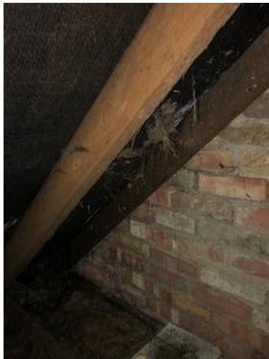
nesting debris noted in torn/sag felt area in loft (building 1)
