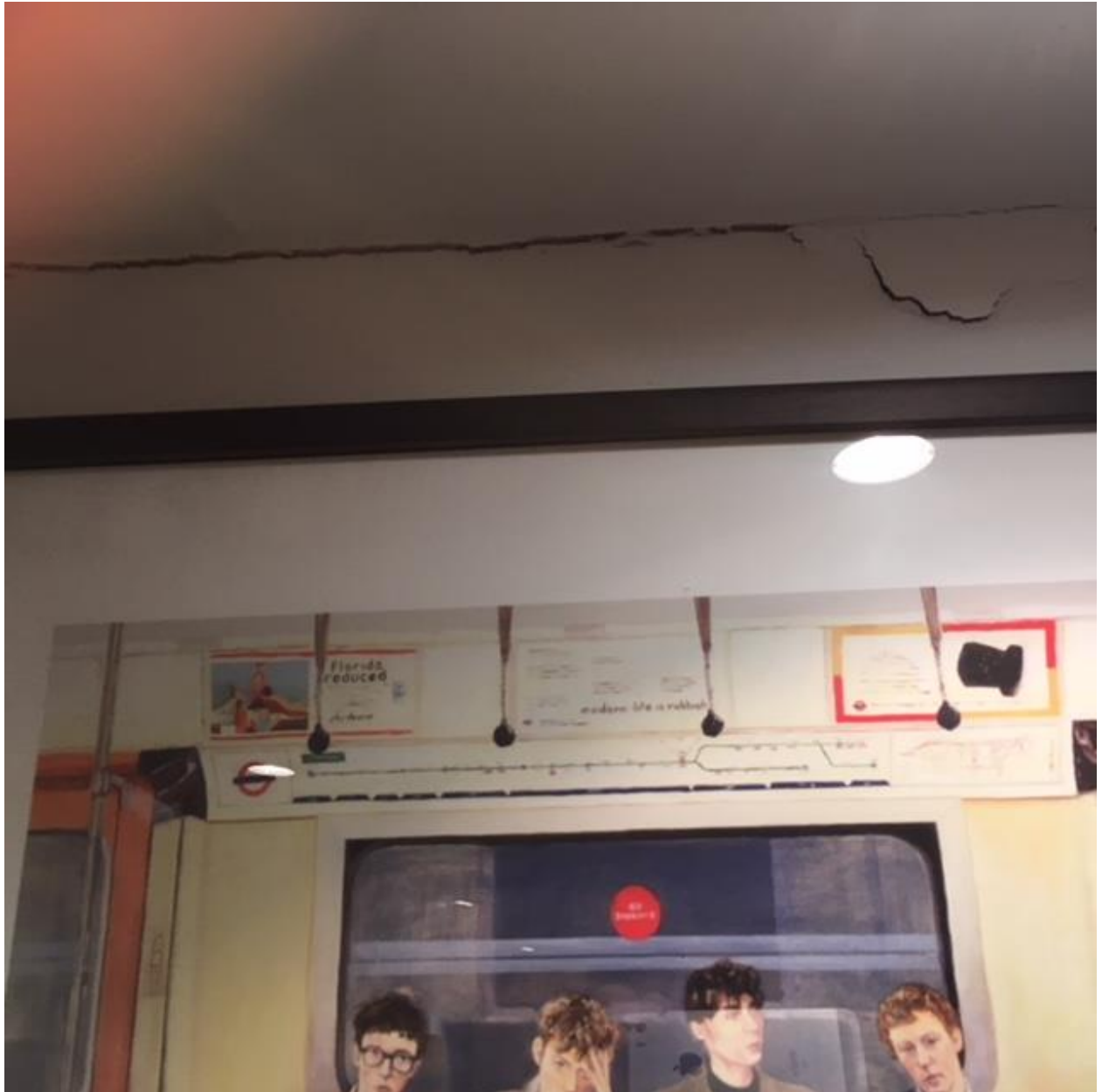
Proof of existing damage at no. 1B Spencer Rise
