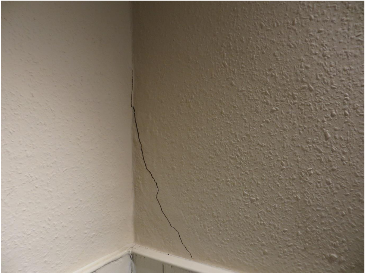
Proof of existing damage at no. 1A Spencer Rise.
