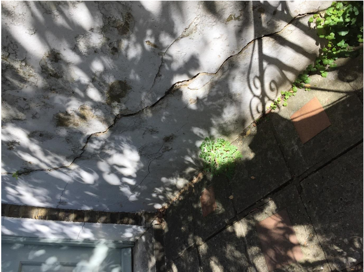
Proof of existing damage at no. 1C Spencer Rise.
