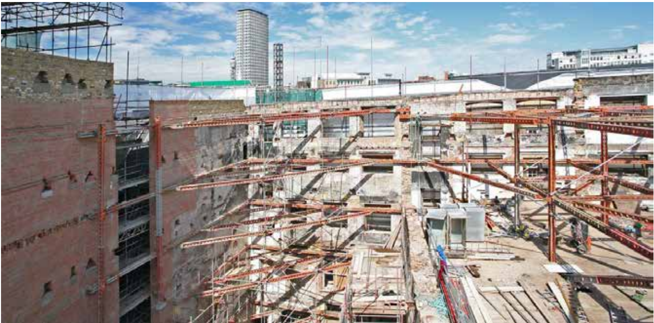
14. Photograph showing the damage to the Seven Dials Warehouse, c.2000 (AKT II)
