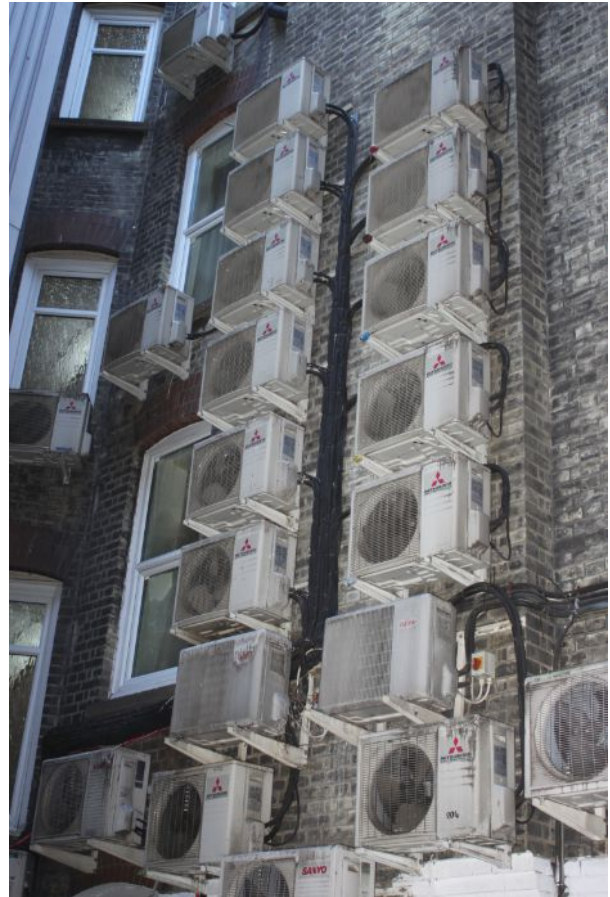
Figure 3: Existing hotel external a/c units
