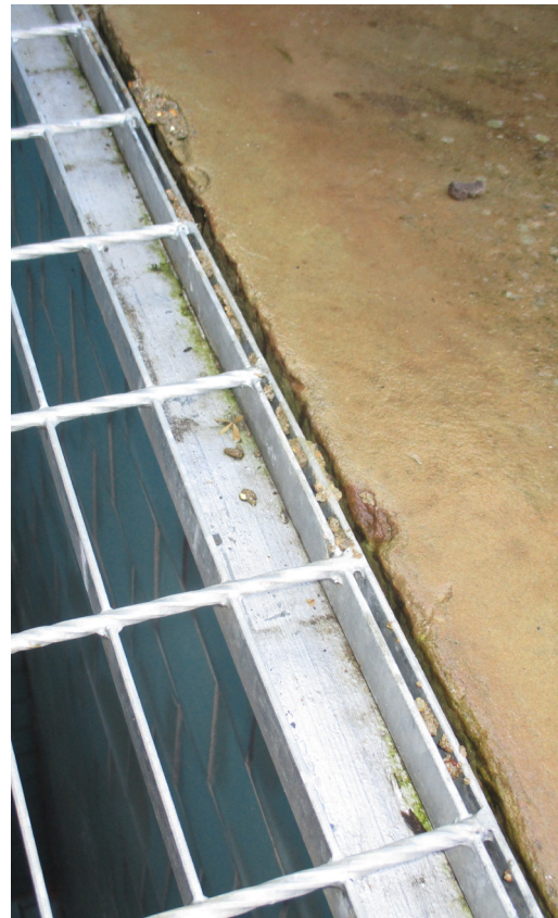
Weak waterproofing point around metal grille over rear lightwell
