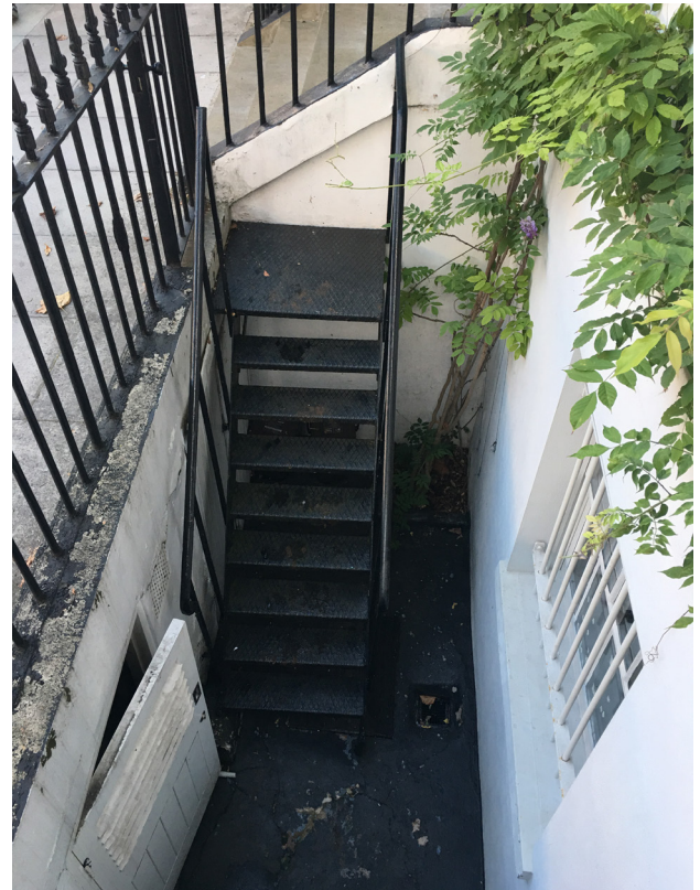
Existing steep, slippery and narrow stairs leading to front lightwell
