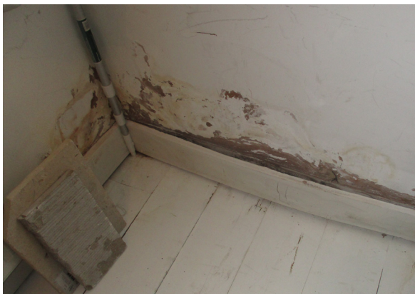
Mains access with blistered asphalted steps (above) Interior damp damage (below)
