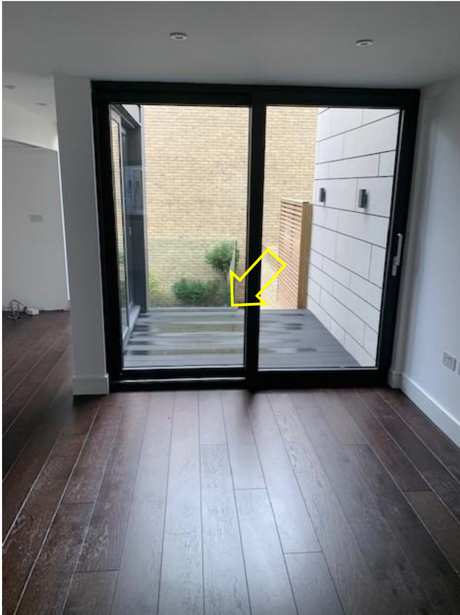
Photo.1 View from within No.17 looking out over terrace towards the garden. Arrow indicates extent of proposed extension.
