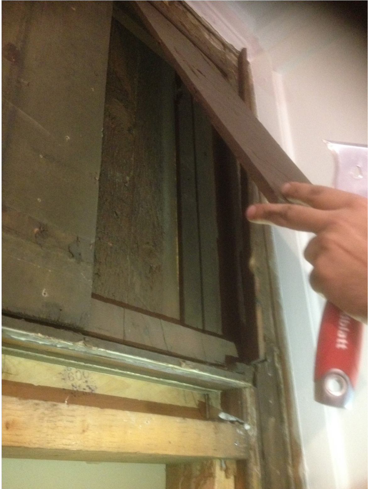
Board lifted to reveal back of full height panelling to Office 7 (now obscured in Office 7 by stud wall added for sound proofing)
