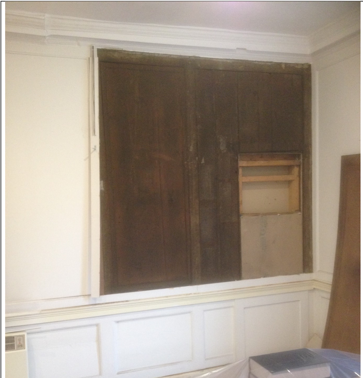
South Wall of Office 8 with planted false panelling above dado removed to show former opening
