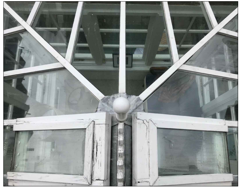
Photo of existing rotten conservatory roof structure
