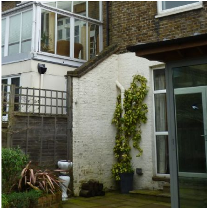
Figure 9: Free standing wall evidence of the original lean-to part of the house
