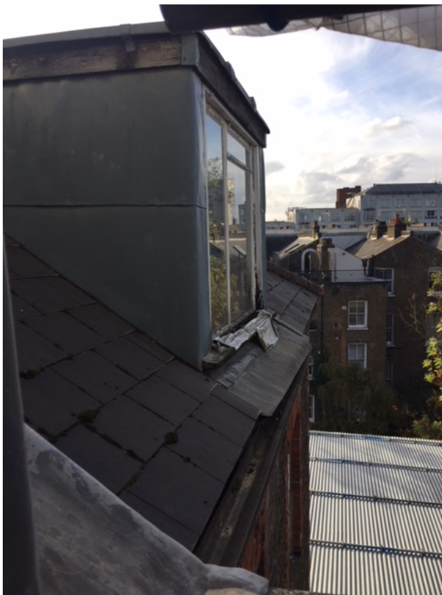
Photo 4 (above): Existing rear dormer at adjacent neighbour No. 148 Fellows Road looking west
