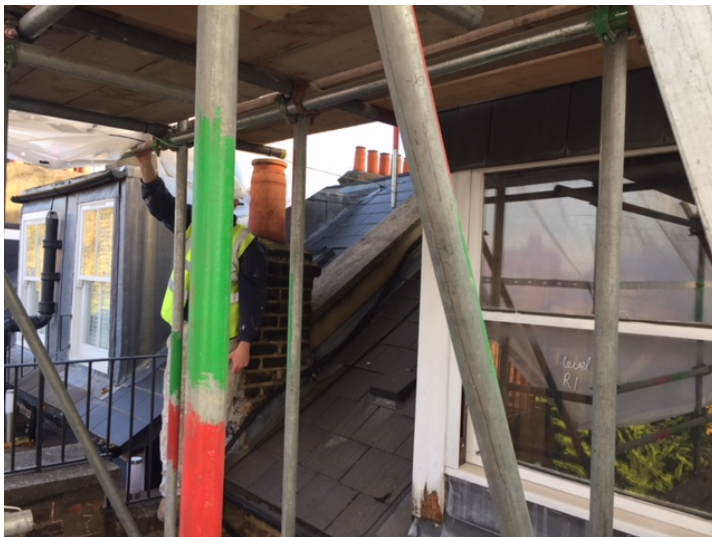
Photo 6 (above): Distance between existing north-eastern dormer window and existing dormer at adjacent neighbour No. 144 to the east
