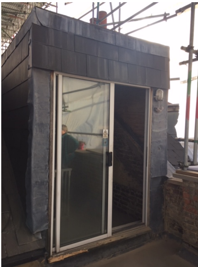
Photo 2 (above): Existing north-western rear dormer adjacent to party wall and above third floor roof terrace
