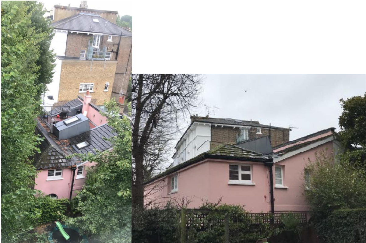
Photo 3 and photo 4: Existing roof of the property and views from the garden of the neighbouring property at no. 6 Albert Terrace.
