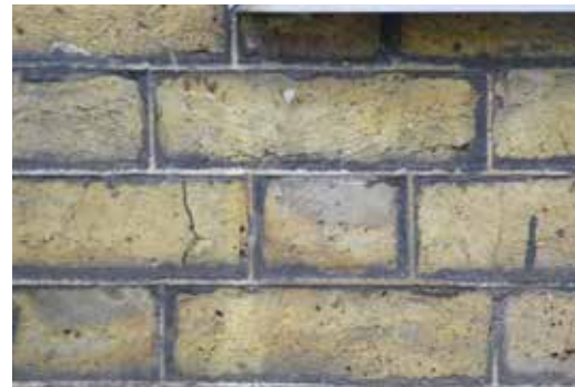
There are some sections of tuck pointing on the front elevation, where this has not been repointed or altered.
