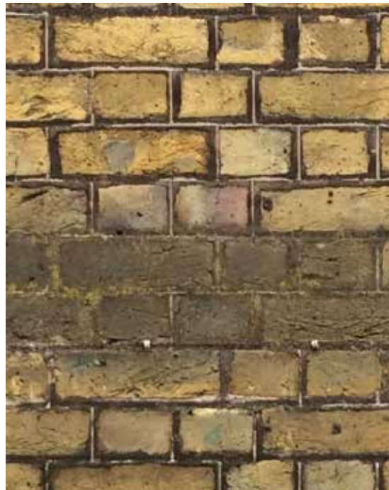
Original lime tuck-pointing has been replaced by large areas of cement-based repointing. The quality and consistency of the pointing overall is poor.
