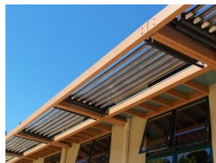
Figure 9: Solar thermal evacuated tubes arranged as brise soleil
