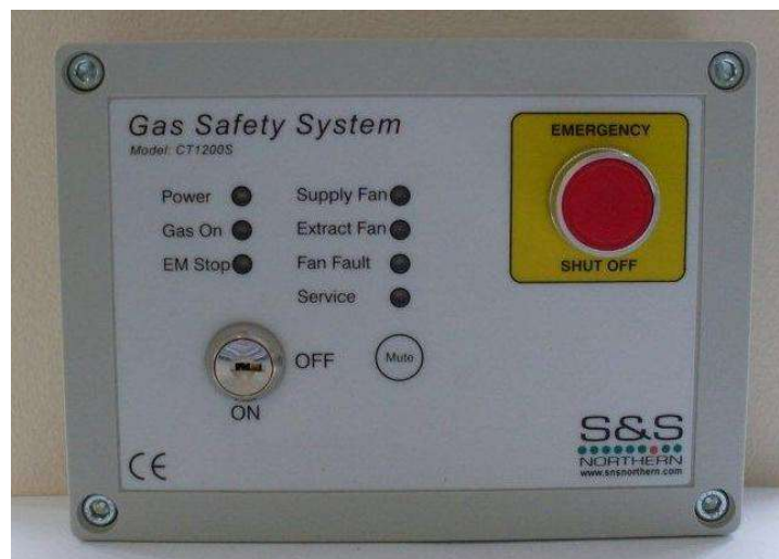
Fig 2 – Typical Gas Interlock Control Panel
