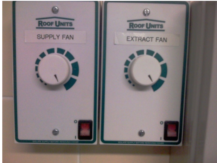
Fig 1 - Fan controls set at full speed (Typical speed controllers shown)
