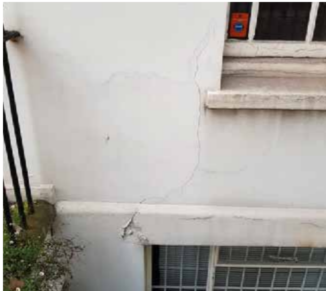
Cracked render on front elevation
