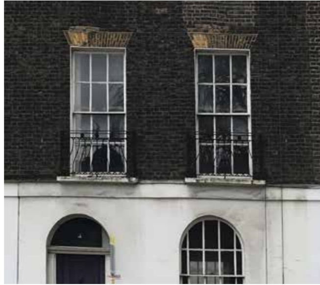
Cracked brickwork to first floor window lintels
