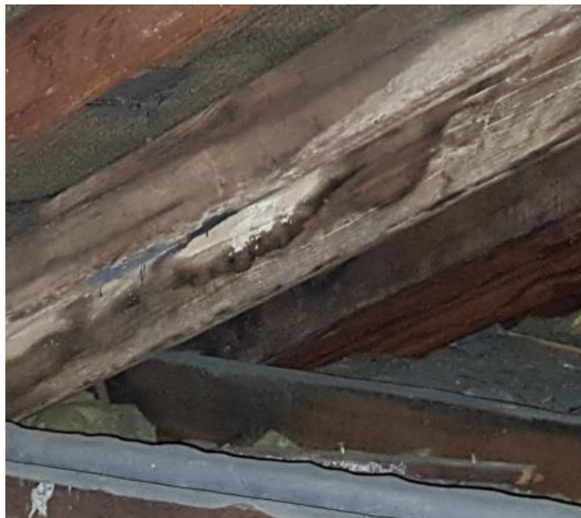
Rot to roof timbers
