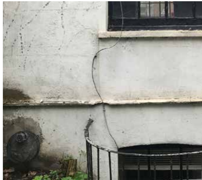
Cracked cement render to rear elevation
