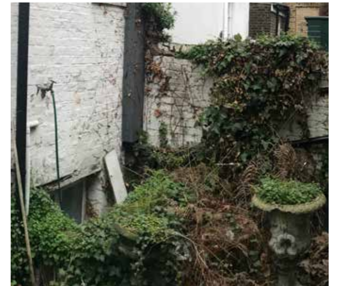
Existing shallow lightwell in rear garden & Boundary wall to no.3
