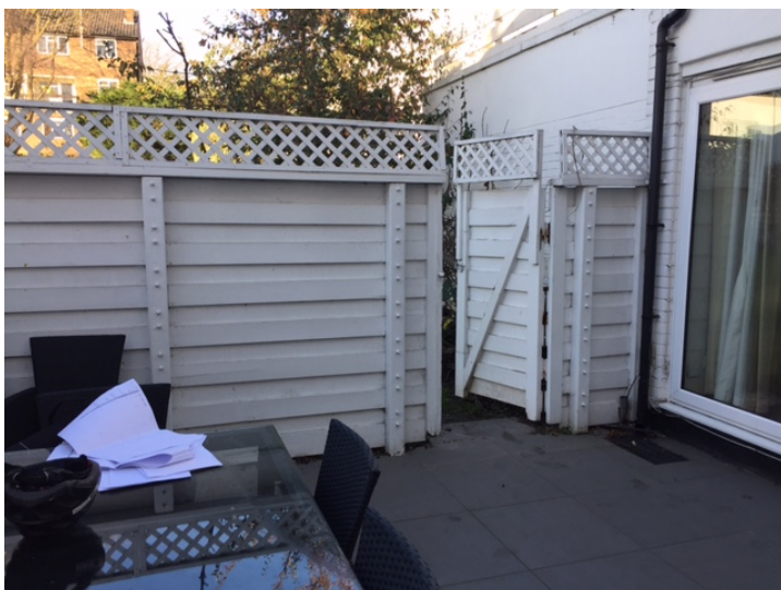
Photo 12 (above): View looking north from rear courtyard of 106 King Henry's Road showing existing rear gate leading to communal rear garden
