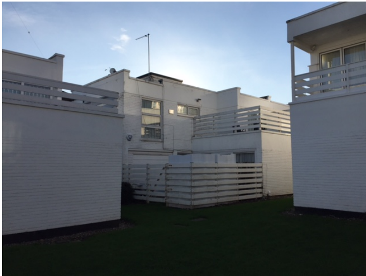
Photo 7 (above): Rear and side elevations of No. 110 King Henry's Road (centre) as viewed from communal rear garden, looking south-west
