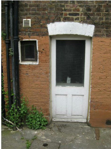
Existing door and window to be replaced with black metal crittall wondows
