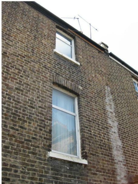
Rear windows to be replaced with timber sash windows
