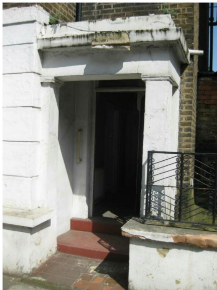
External repairs and decorations required
