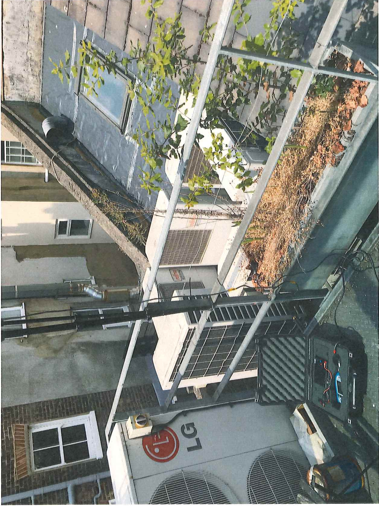
Photo D – Existing Condensers on Roof Area of No.3 Bromley Place (Units not Operating)
