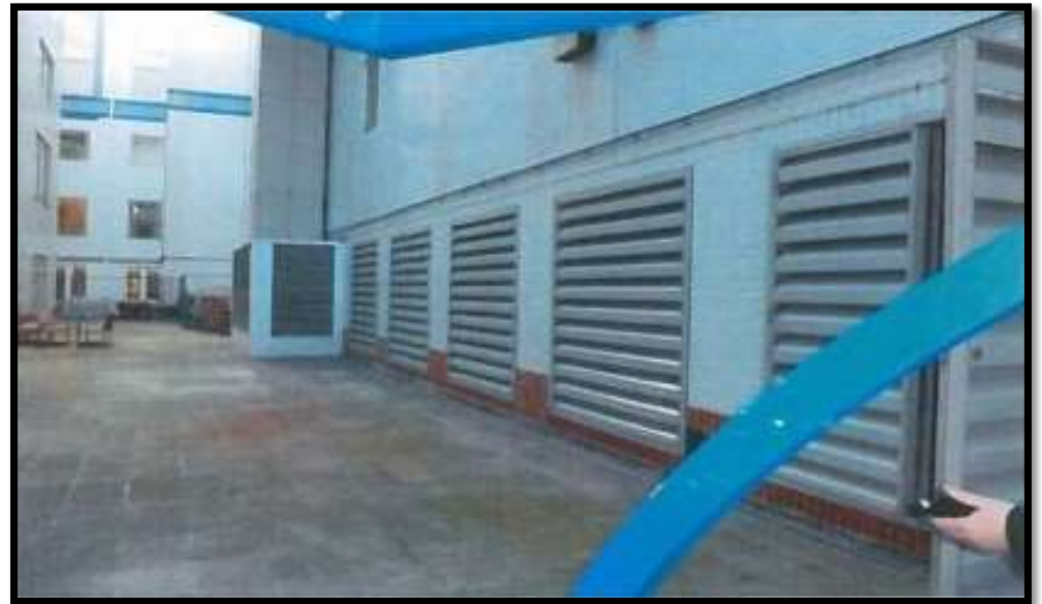
FREEMASONS' HALL PROPOSED LOCATION FOR STAND BY GENERATOR
