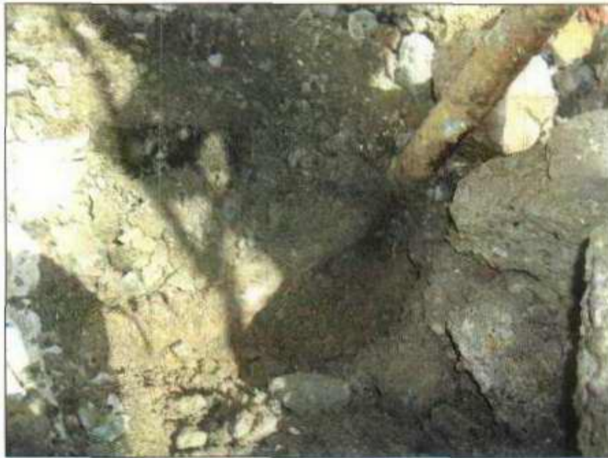
Photo 4. Pipework from under the re-fuelling point
