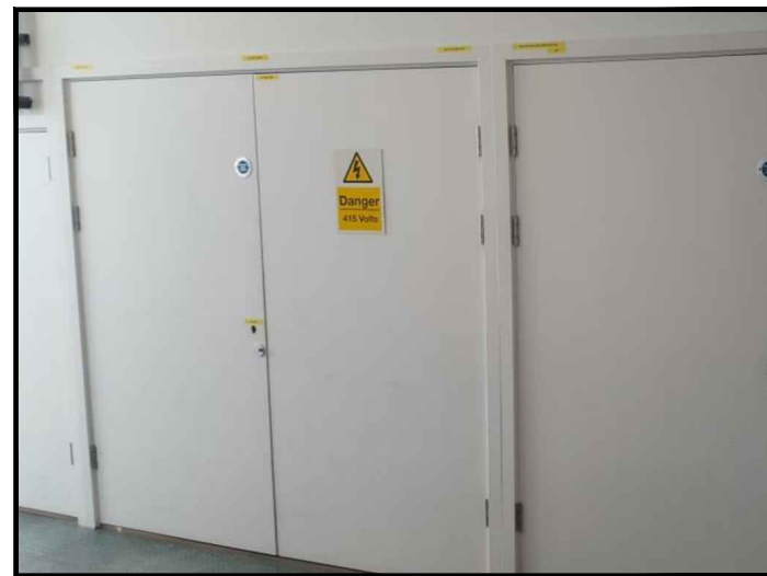
EXISTING LANDLORD DISTRIBUTION BOARD
