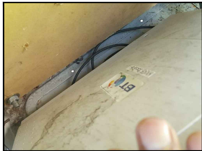
EXISTING BT FIBRE TERMINATION POINT
