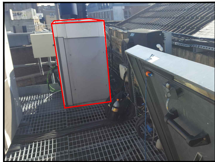
EXISTING CABINET TO BE DE-COMMISSIONED
