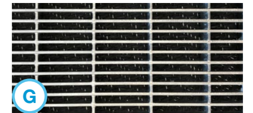
G Open metal cover to davit plinths at L05
