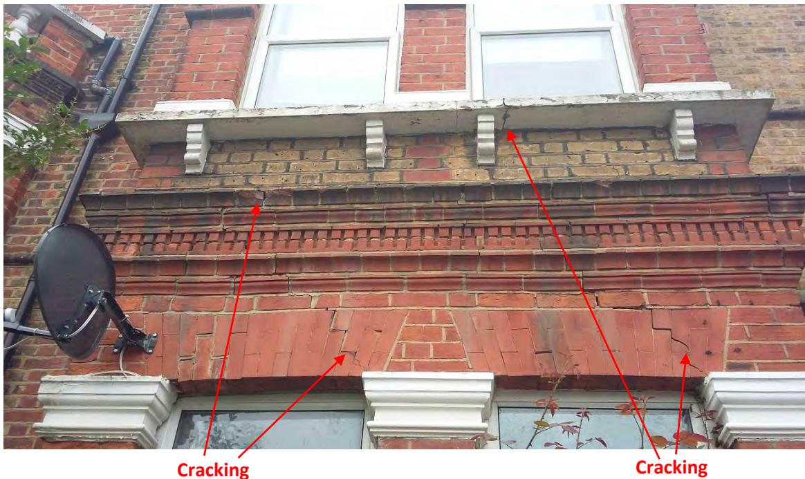
Photo 2: View of the front bay of No.8. Extensive crack damage is visible around the windows of the front bay, including in the side windows (not visible here).
