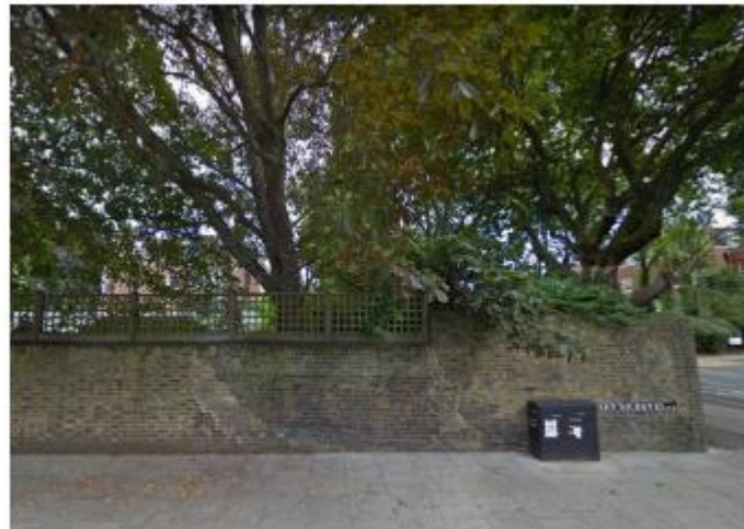
LOCATION B WITHOUT POLE
