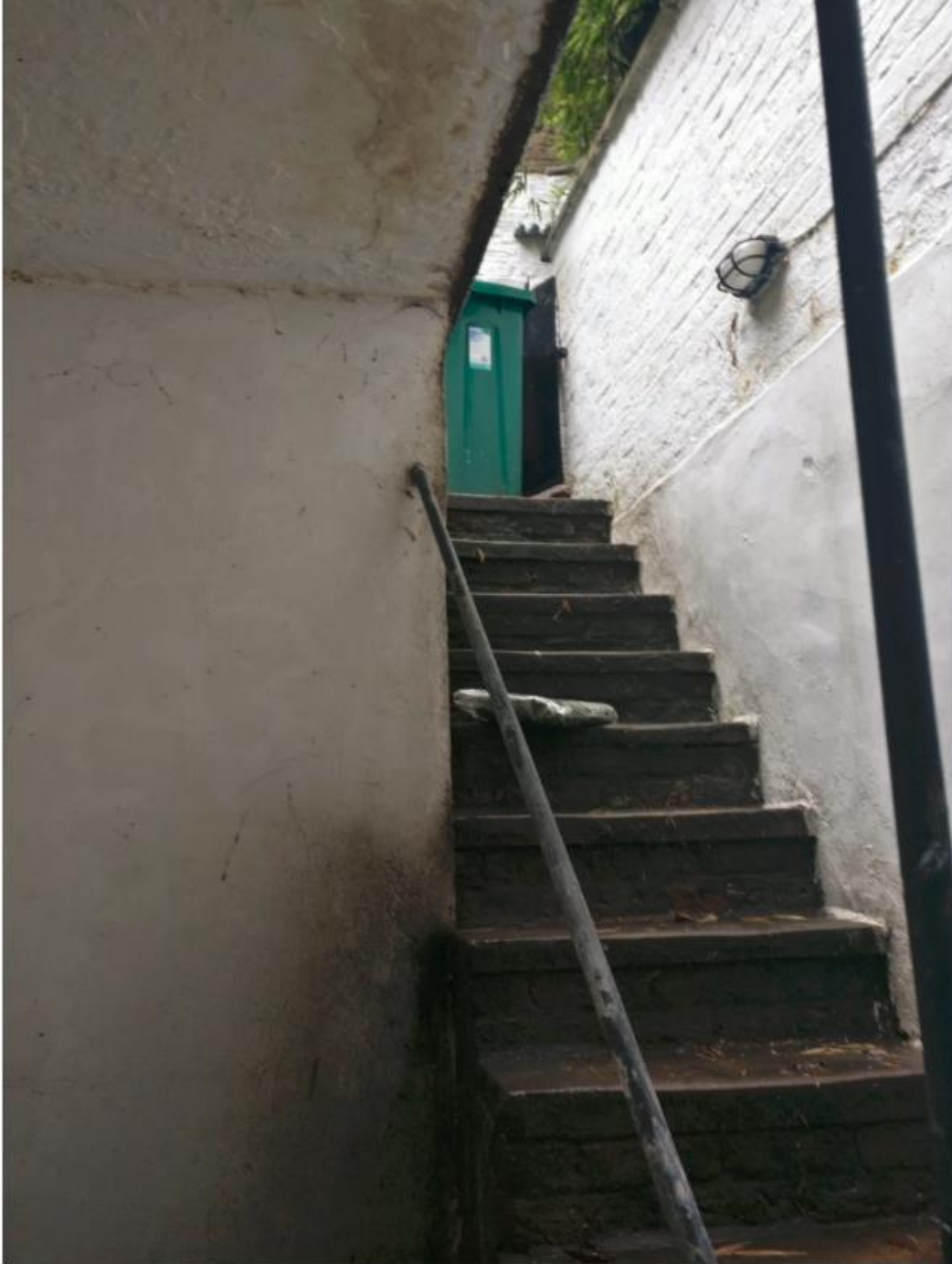
View of basement floor level staircase up to ground floor level (wall and area alongside staircase to left in photo to be removed)
