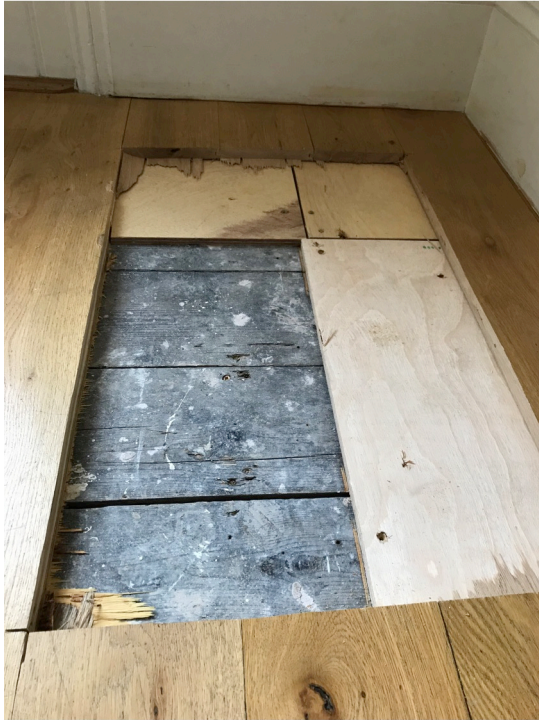
Ground Floor- Existing Floor Materials- 18mm non-original floorboards, 12mm plywood, older floorboards
