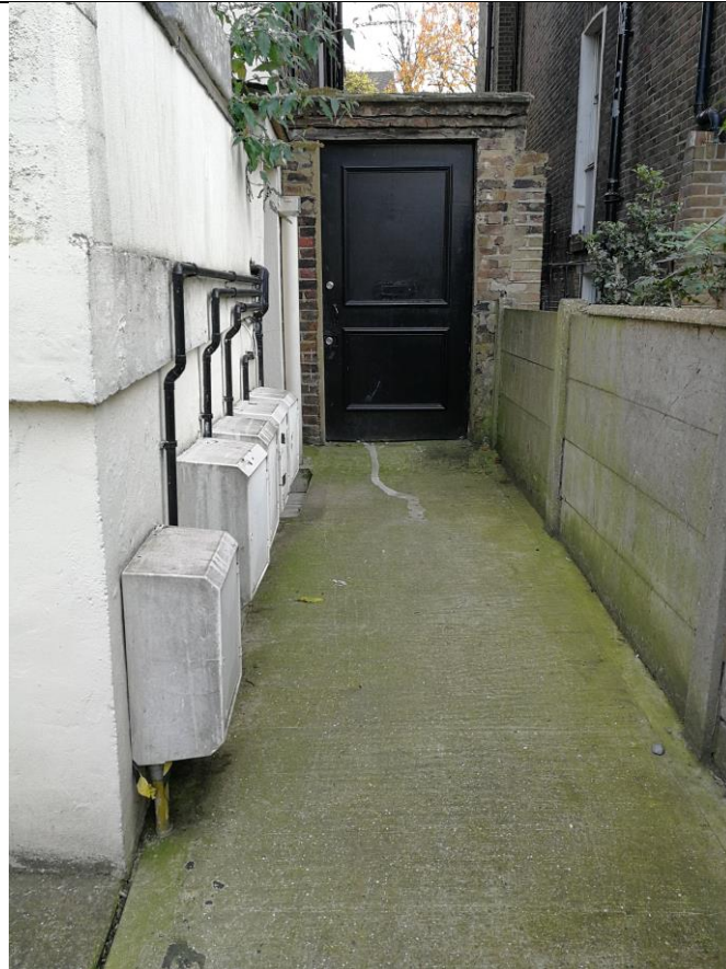
Photo 6 – Right flank wall of entrance steps. External gas meters.
