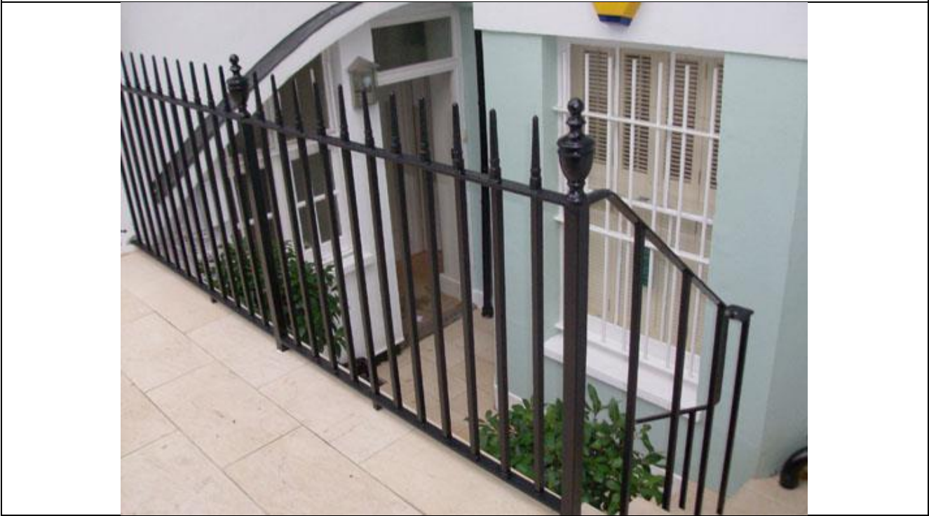
Photo 9 – Proposed railings detail for the perimeter of the small flat roof over the entrance steps
