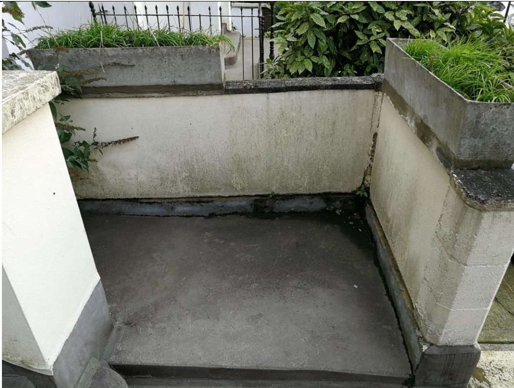
Photo 7 – Section of flat roof to the right hand side of the entrance step. Blockwork parapet wall detail.
