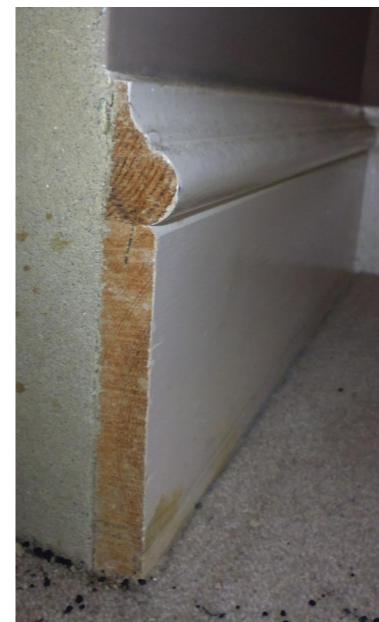
Existing skirting from room 3.03
