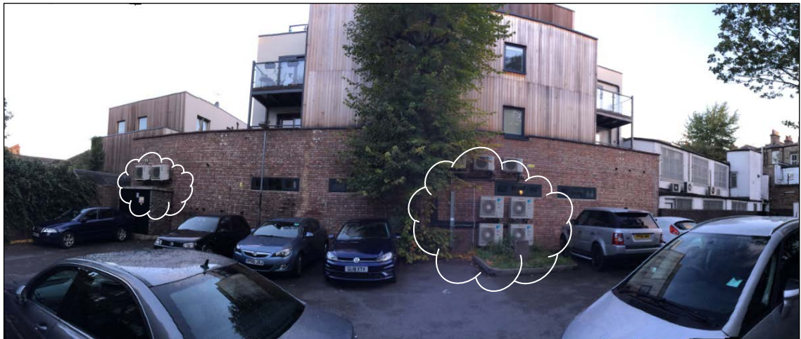
Figure 2.2: Installed Air Conditioning Condenser Units
