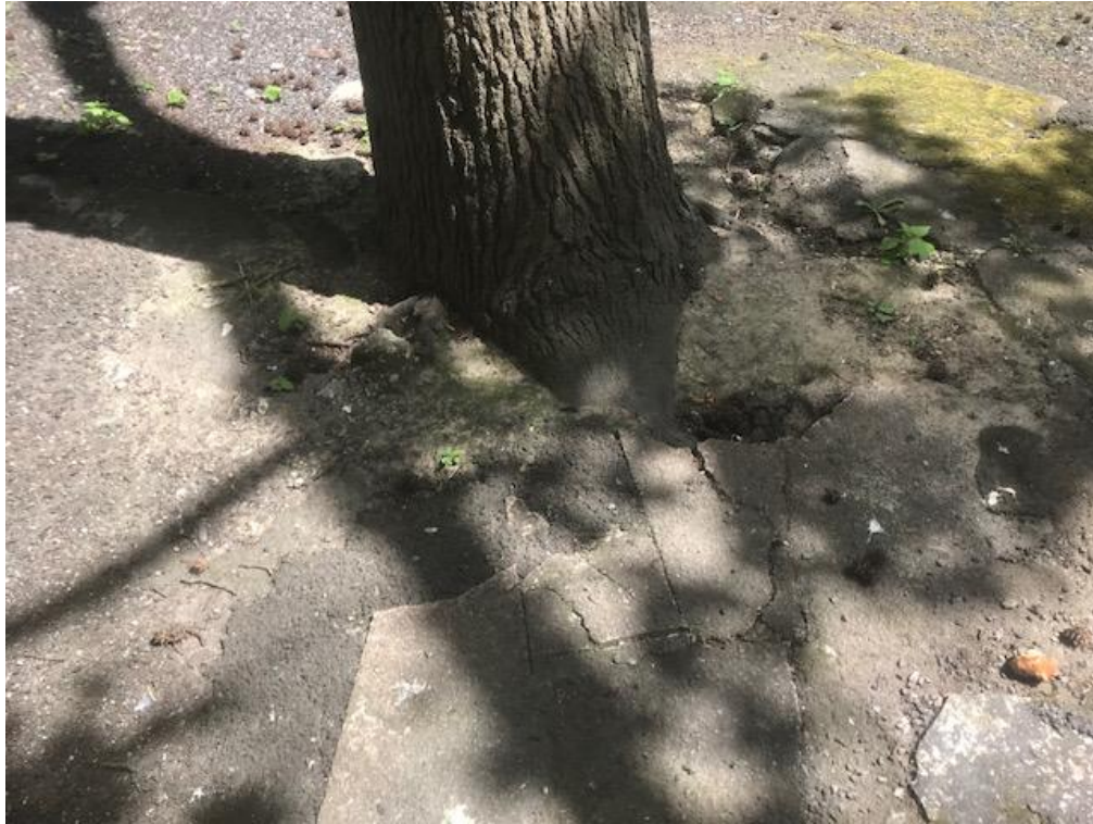
Photograph 5 – T2 roots lifting tarmac. No permeable rooting zone.
