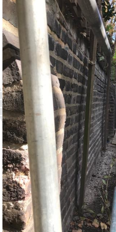
Right: Deflection to north (rear) boundary wall.
