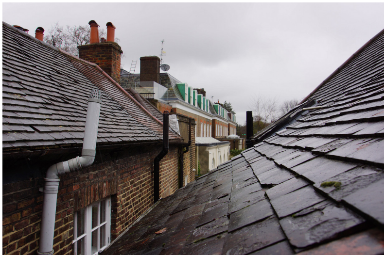
The existing roof clay tiles are at the end of their serviceable life and need replacing. The waterproof layer beneath is plastic and not breathable, which results in condensation building up on the structure beneath. This needs to be replaced with a breathable membrane.
