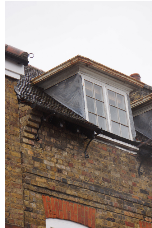
Dormer cheeks and mouldings are in a poor state of repair and need remedial work.
