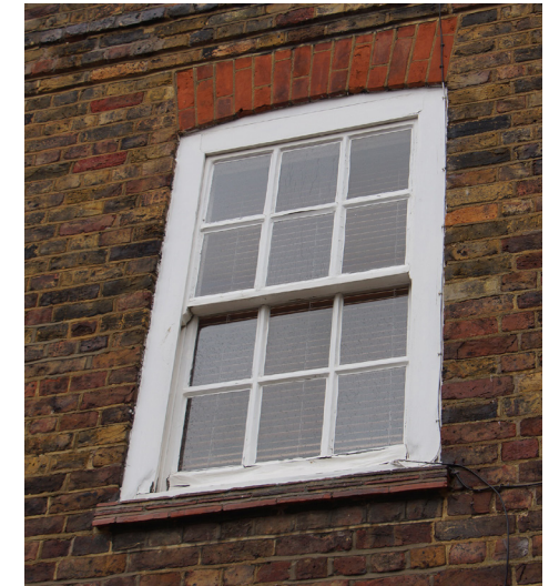
Some of the windows are rotten and need repairing and redecorating to make good.
