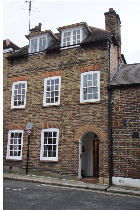
Front facade and entrance. Mortar has come loose and needs to be repointed.
