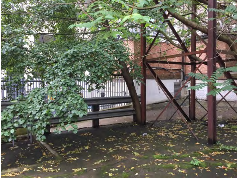
Photograph 5 – Tree T2 growing next to steel frame.
