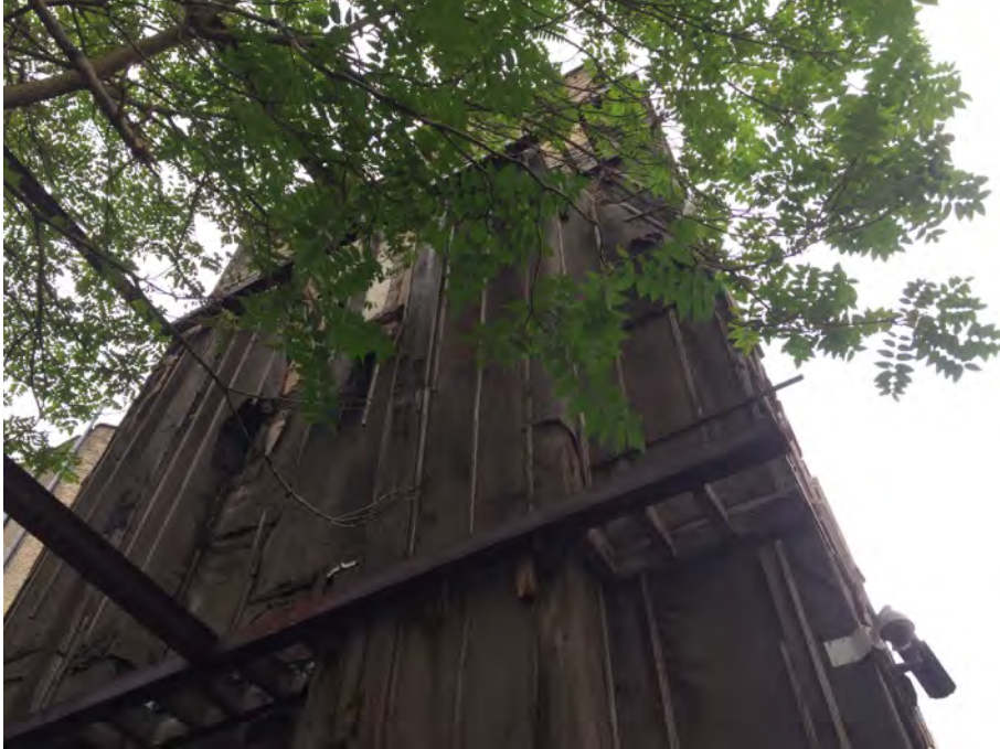
Photograph 9 – Limbs from T1 contacting derelict building.
