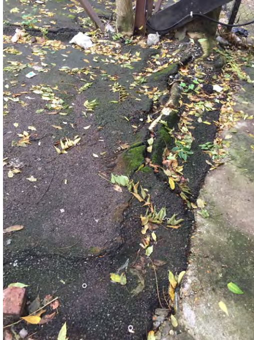
Photograph 7 – Damage caused to tarmac by incremental root growth.
