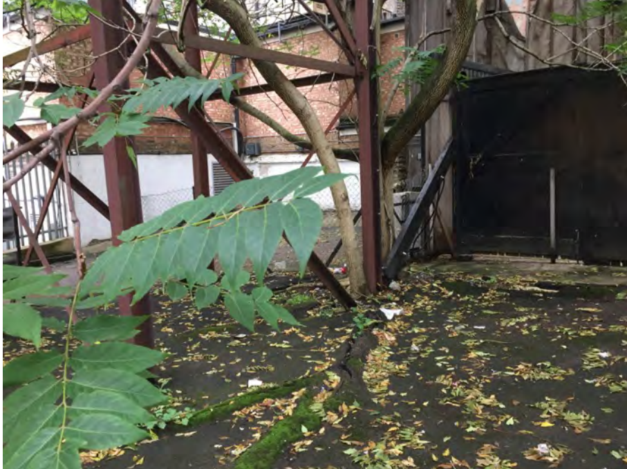
Photograph 3 – Damage caused to tarmac by T1.
