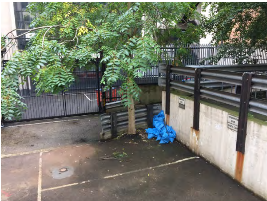
Photograph 4 – Damage caused to tarmac by T3.
