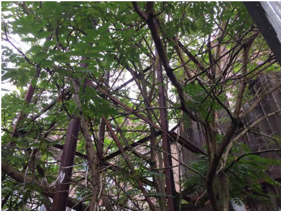
Photograph 6 – Tree T1 growing through steel structure.
