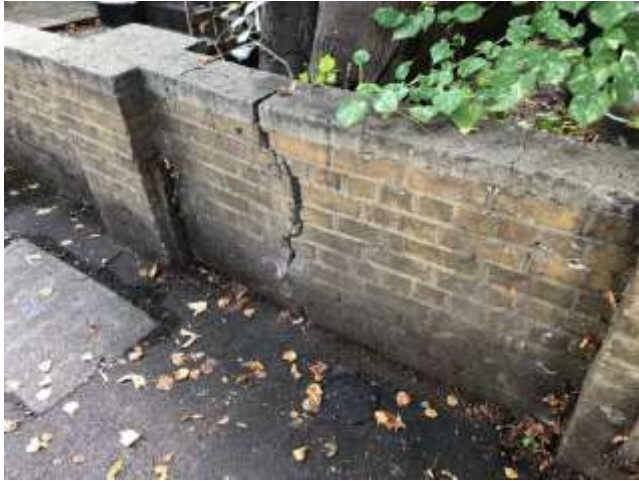
Damage to wall
