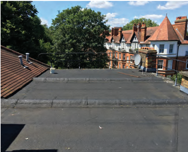
Photograph of the existing roof showing the uneven surface.
