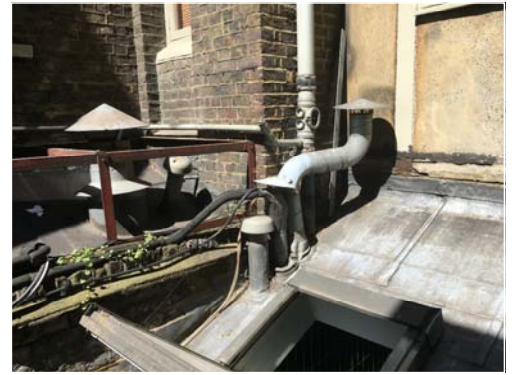
Existing extract ducts to be removed shown exiting through ground floor roof of No.55.
