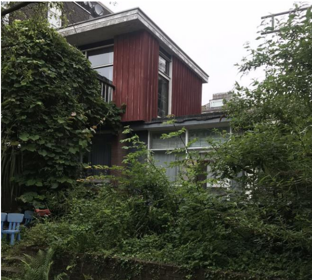
View of the back elevation to the rear garden. The late 1960's extension can be seen, with its poor combination of materials and composition.
