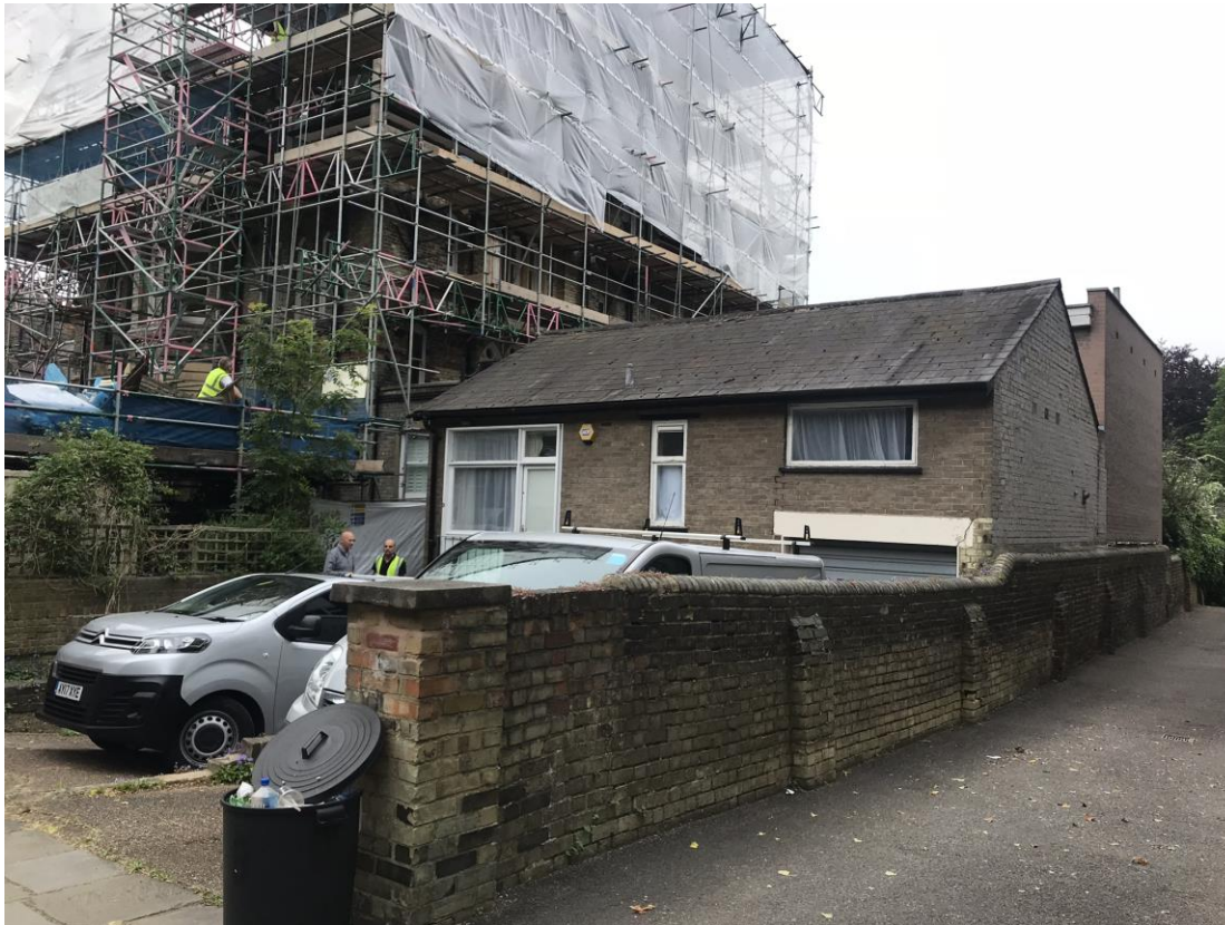
View of the application site. The late 1960's rear extension can be seen on the right hand side.
