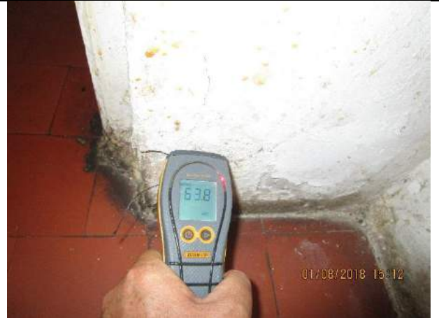
High levels of 63.8% moisture were recorded to the lower areas of the walls as indicated
