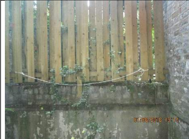
High rear external ground levels abutting the walls
