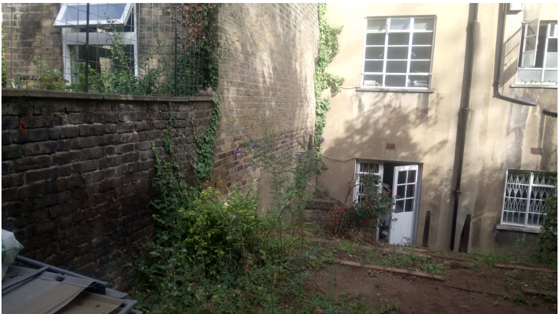
View of the party wall and the neighbouring property (to the left)
