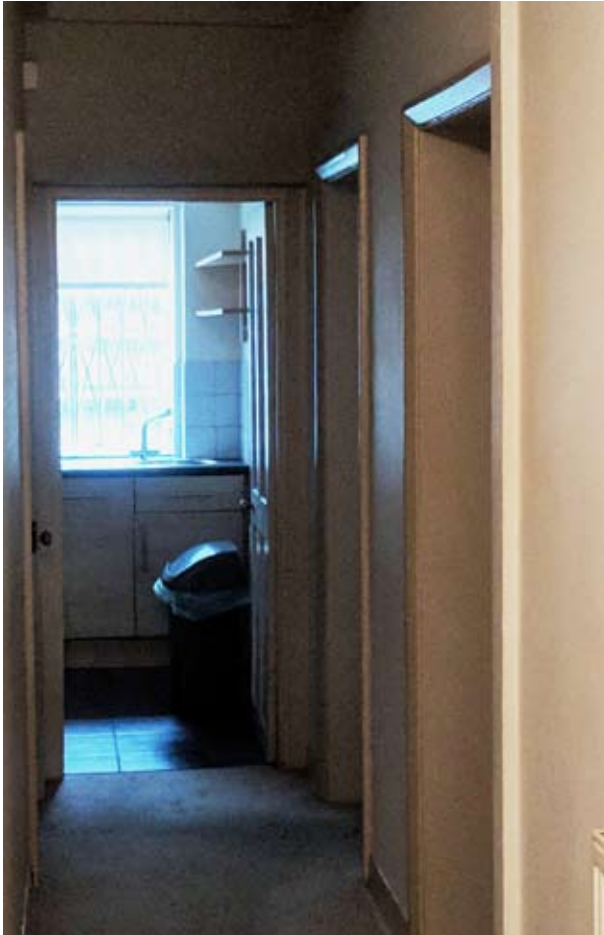
Fig. 16 Existing door, threshold & wall surround to be knocked through to insert full-height slim-framed fixed glazed screen (between hall LG01 and kitchen LG05)
