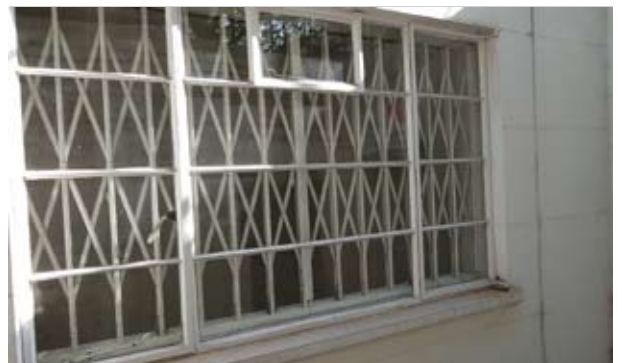
Fig. 14 Existing steel window to be replaced (external view)
