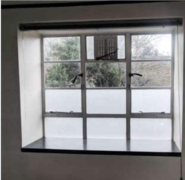
Fig. 20 Existing steel window to be replaced with new crittal-style window (Bathroom UG03)
