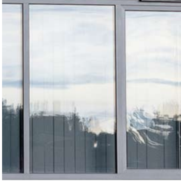
Light-grey aluminium windows and doors to the extension (bedroom window, dining room doors)
