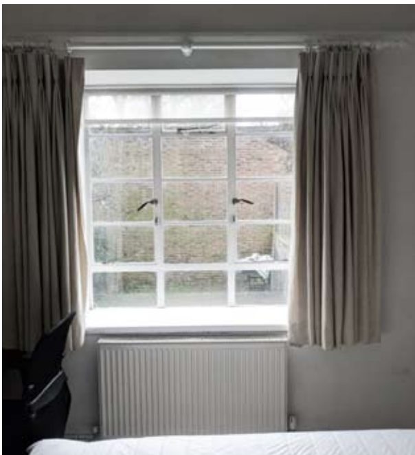
Fig. 22 Existing window removed, wall below cill knocked-through to form threshold to new extension (UG04)
