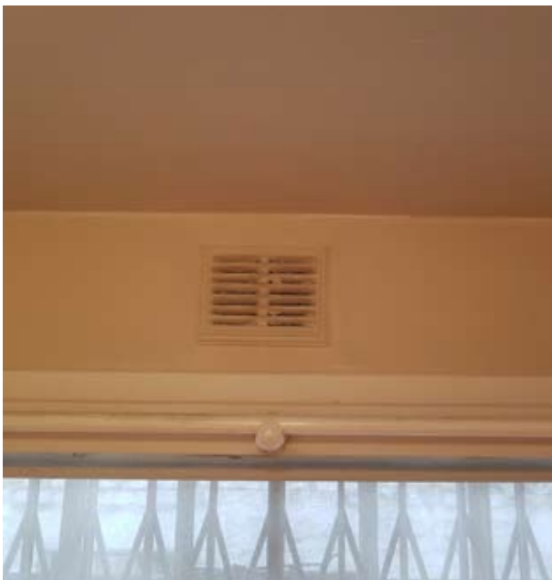
Fig. 12 Existing ventilation grille to be removed and filled. Finished internally with plaster to match existing - LG02 (internal view)
