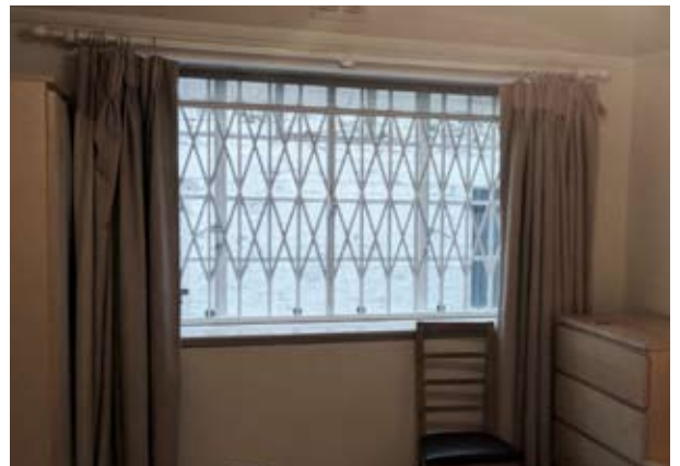
Fig. 15 Existing steel window to be replaced to reception room LG02 (internal view)
