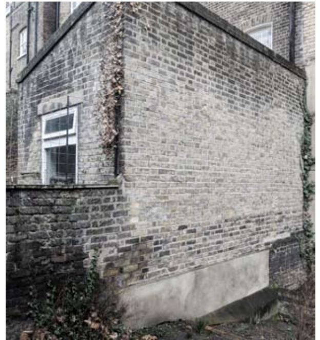
Fig. 23 Existing corbelled foundation to neighbouring extension to be protected fully during works and retained.
