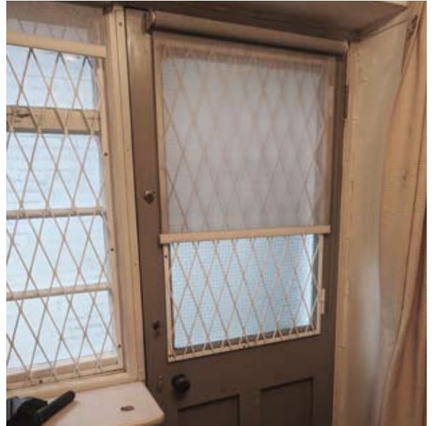
Fig. 13 Existing front door and sidelight window to be replaced to hall LG01 (internal view)
