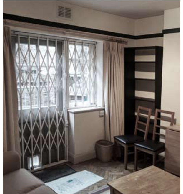
Fig. 17 Existing door and sidelight removed, wall knocked through under window cill. Vestigial wall nib to right-hand-side of opening retained (LG04)
